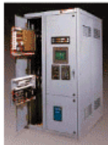
Automatic Transfer Switches
