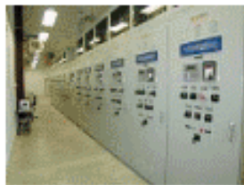
Digital Paralleling Switchgear
